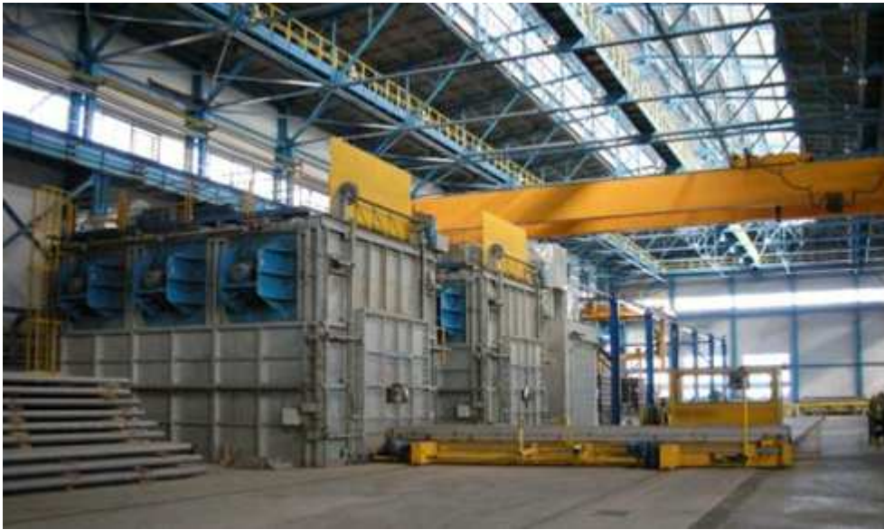
Fig. 4: Example of a typical billet homogenising system consisting of two batch furnaces and a cooling chamber (Otto Junker design, as in the following photos)
