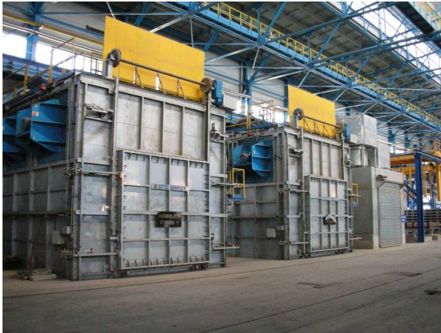
Fig. 3: Discontinuous (batch-type) homogenizing plant with cooling chamber, designed by Otto Junker
